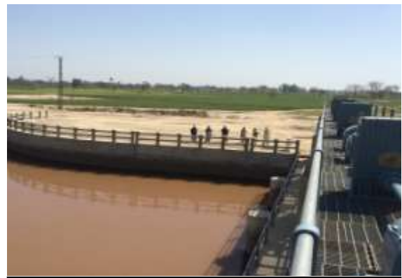
Photograph No. 4: View of the newly constructed cross regulator through temporary occupation of private land at LBDC main canal.
